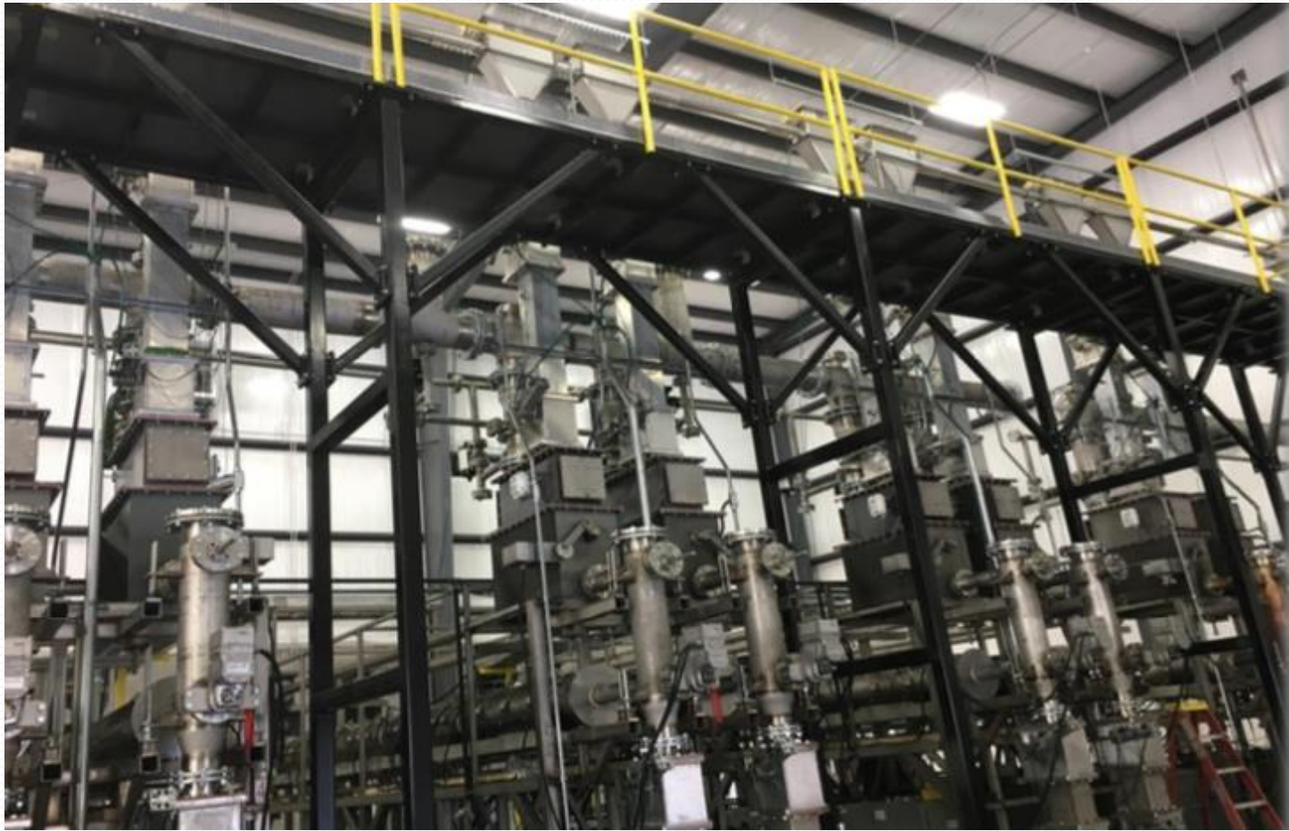
Pyrolysis Unit Installation 24 units, each with two Pyrolysis Tubes Capacity per unit: 10.5 tons/per day
